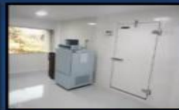
Cold Room (Outer View)
